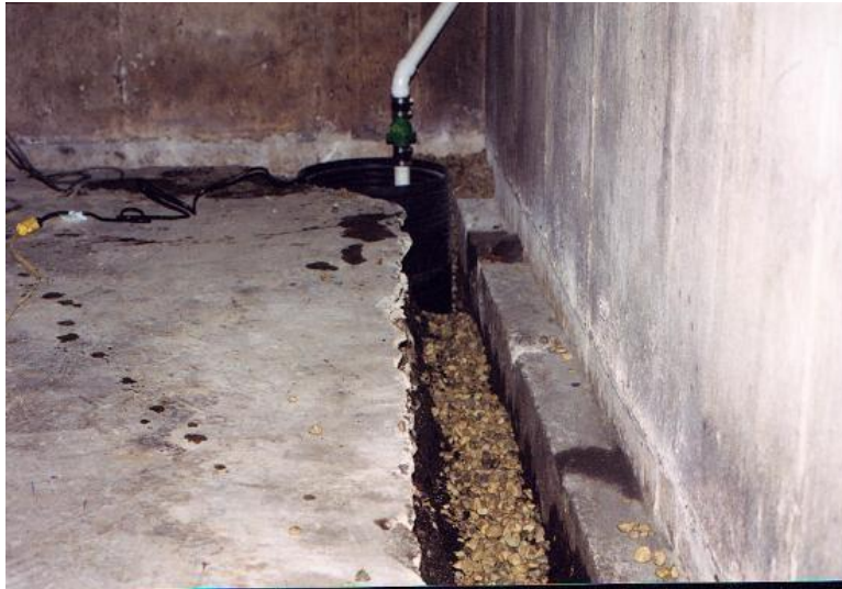
Figure 1 – Interior Foundation Drainage System with Sump Pump
