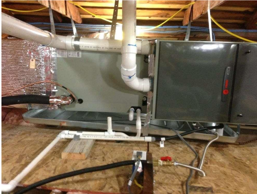
Figure 4 - High-efficiency gas furnace in an attic space. Note large-diameter PVC pipes used for combustion air and exhaust gases.
