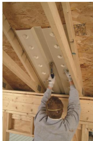
Figure 5 - Attic vent chute installed in each cavity between adjacent rafters/trusses. These are installed continuously from the vented soffit to the ridge/gable vent to allow cooling of the roof deck.
