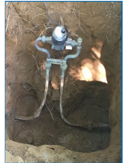
Example of Meter Pit Source: LSLR Collaborative 2018
