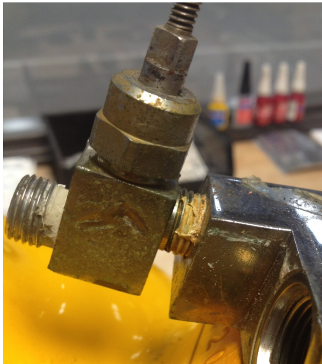
EGS valve body damaged, some sort of plumbers putty on connections
