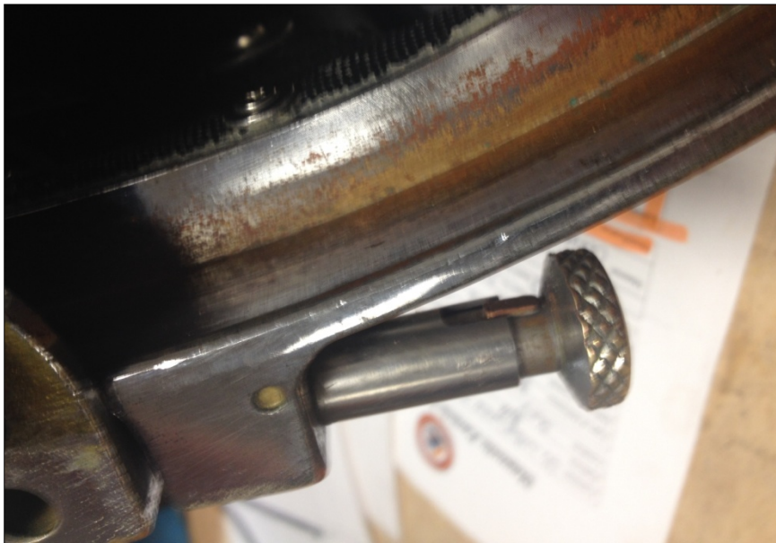
Both pull-pins sticking, and difficult to push or pull; in need of repair
