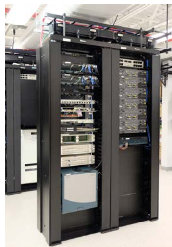
2016 Telecom Phone Switch
