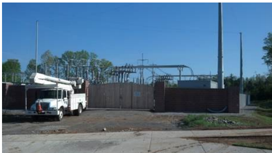
South West Substation
