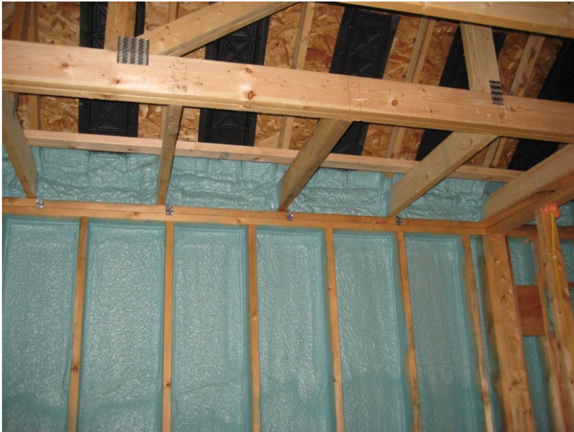
This is completed sprayed polyurethane foam (SPF) insulation. Photo courtesy NCFI Polyurethanes
