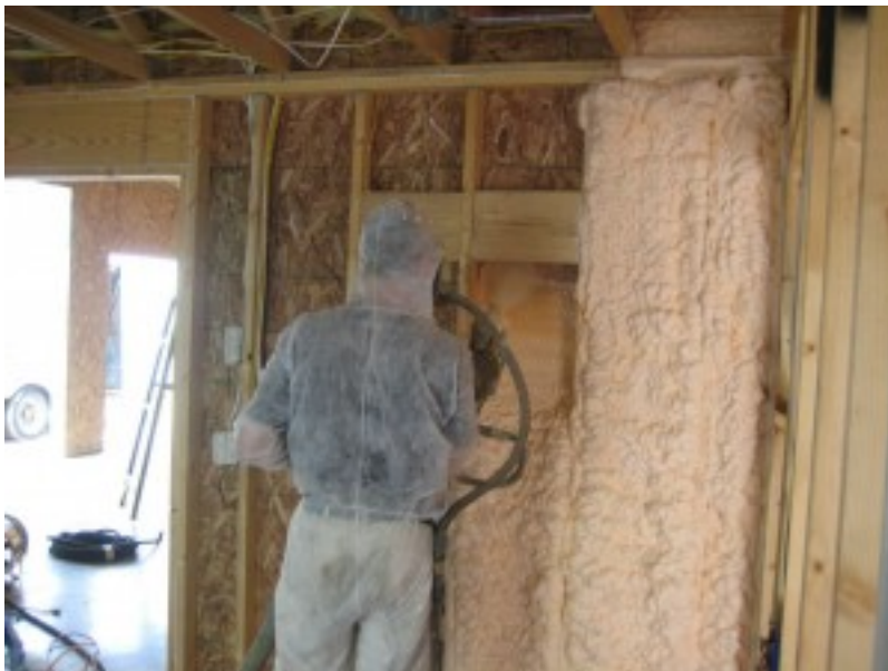
This photo shows the application of SPF below a steel roof deck. Photos courtesy Gaco Western
