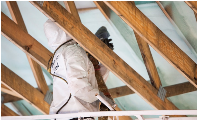
Installation of spray polyurethane foam under the roof deck to create an unvented attic. Photo courtesy of Honeywell.
