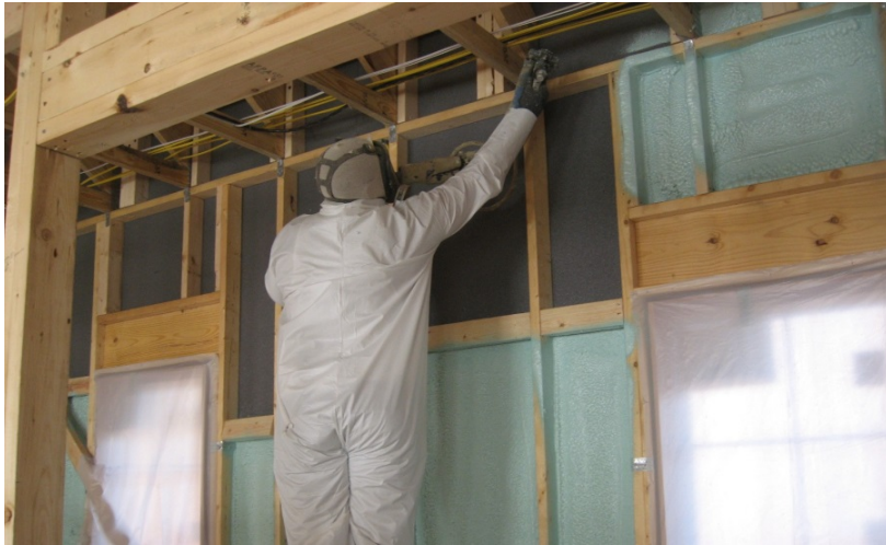
Installation of closed-cell spray polyurethane foam over expanded polystyrene (EPS) sheathing to create a high performance wall. Photo courtesy of BASF.
